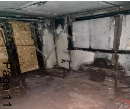
Fire Ignition Point Battery Hoover
